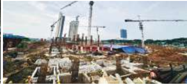
Ongoing construction works of Jakarta Premium Outlets® is on track to complete by first quarter of 2025
