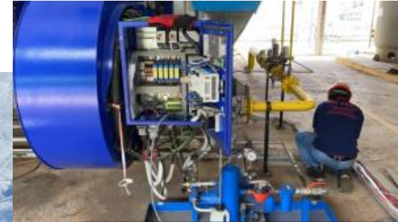
Commissioning of burner - Aug'20
